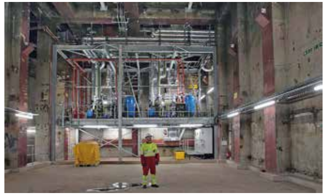
The turbine hall. Photo Martin Godwin
